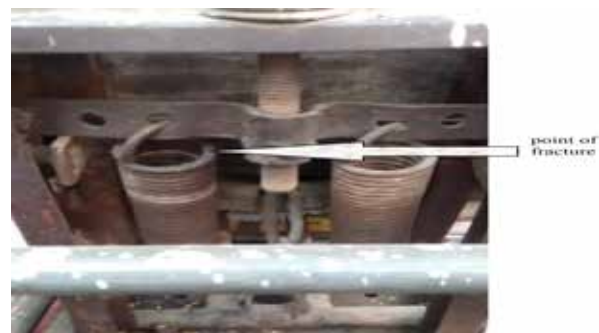
Figure 1. Point of Fracture of Existing Spring
